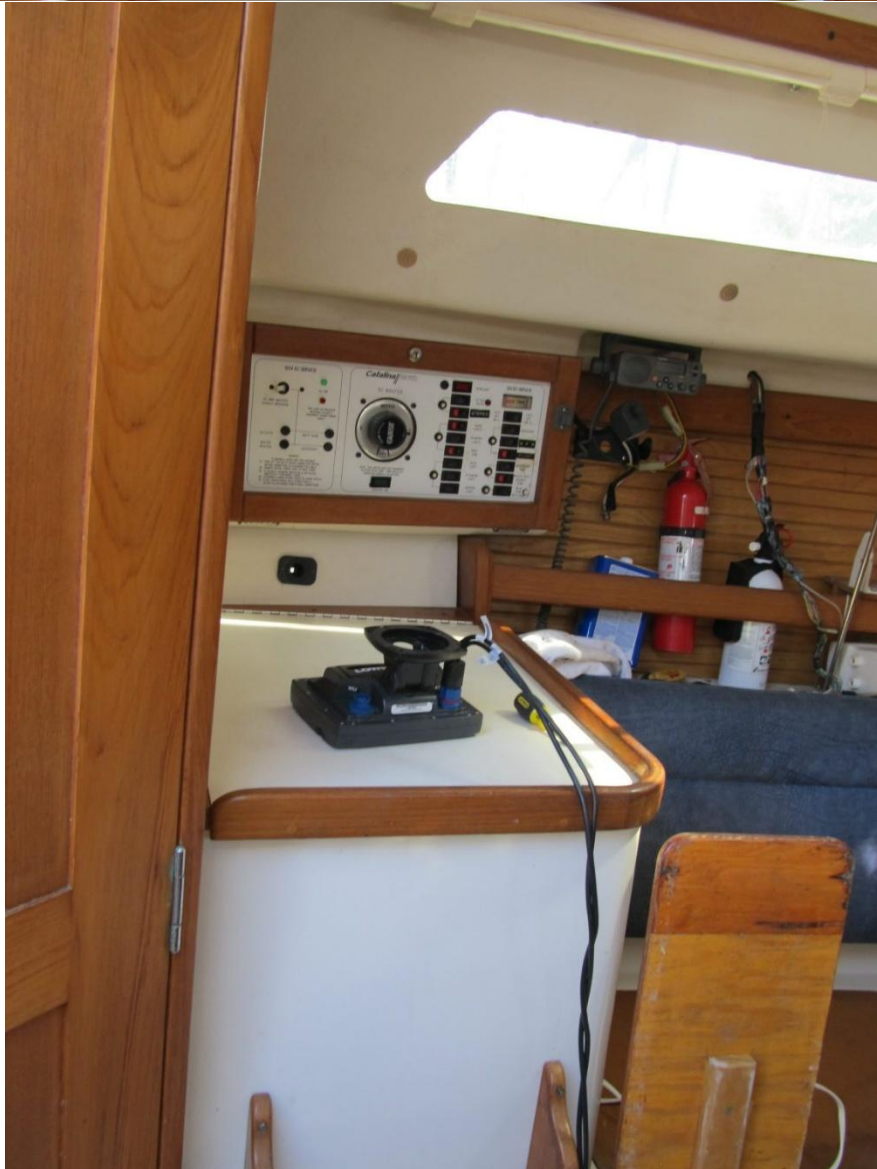
Electrical panel, ice box, and fire extinguishers.
