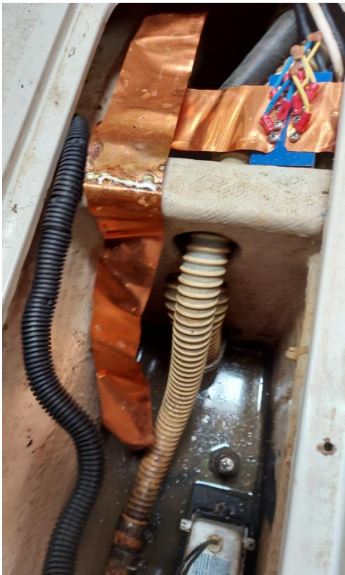
Hull grounding for "Witches Broom" masthead lightening protection and bypassed for ham radio aboard.
